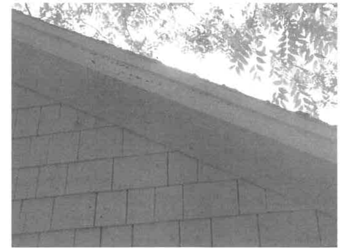
INSECT DAMAGE ON GARAGE RAKE AND SHINGLES.
