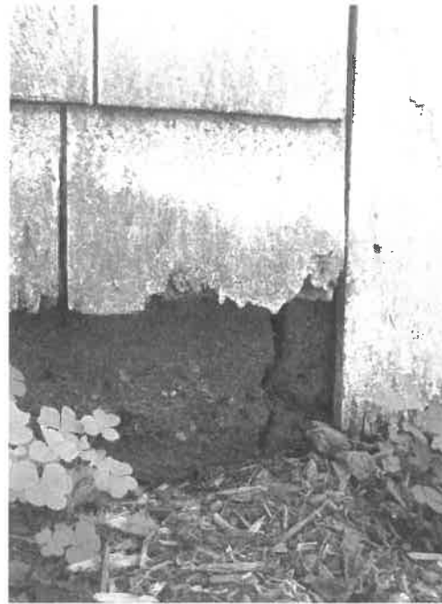
ROT ON GARAGE SHINGLES AND CORNER BOARD.
