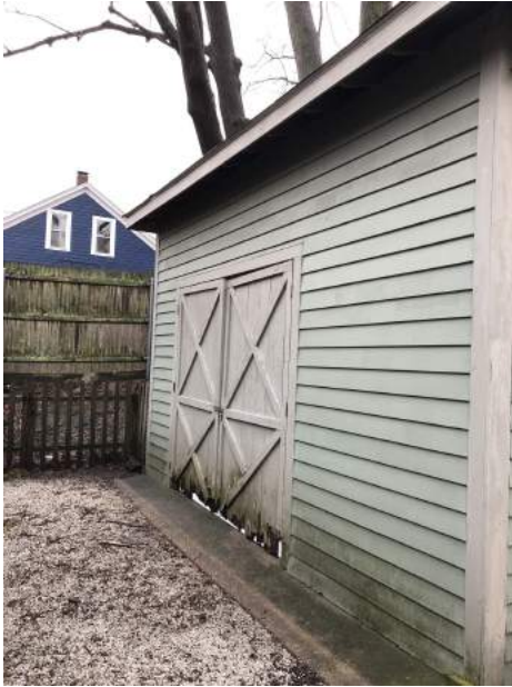
North Side (deteriorating doors)
