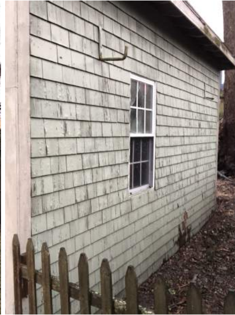
South Side (broken window)
