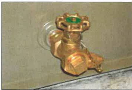
Figure 3. Drain valve with sampler.
