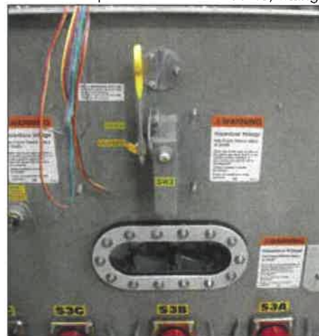
Figure 8. VFI transformer with visible break.
