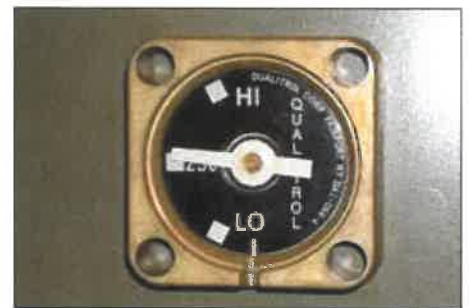
Figure 5. Liquid level gauge.
